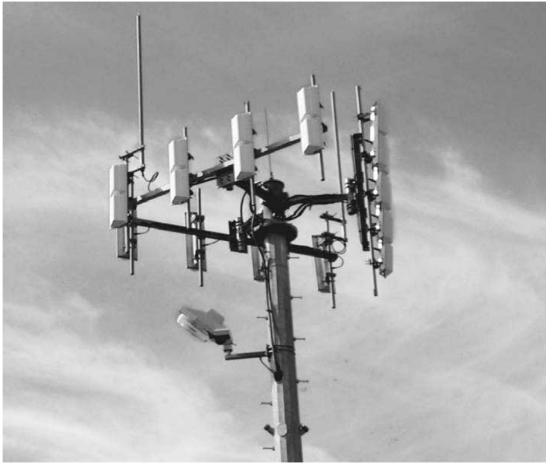
Figure 4.23 Triangular array of dipoles used as a sectoral base-station antenna for mobile communication.
